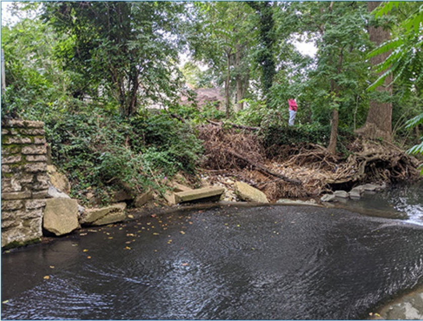
Erosion along Lubber Run impacting mature tree canopy.
