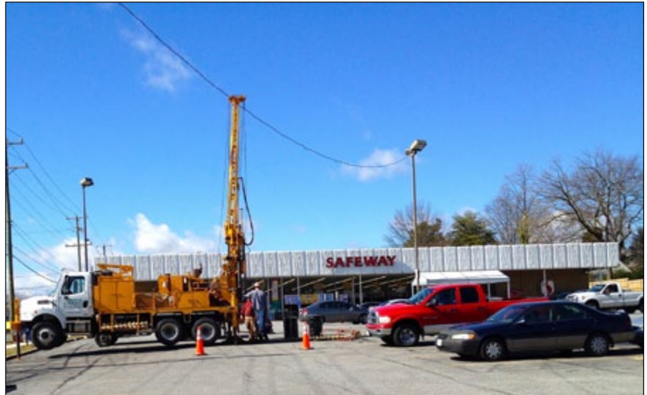
Connolly & Associates Drilling Services obtaining soil samples at Bluemont's Safeway in Feb.
